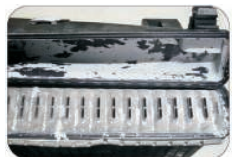
Evidence of aluminium oxide residue settle inside the tank.
