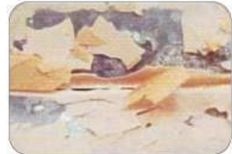
The header plate and inside the tube are covered with brown residue
